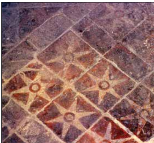
Encaustic (inlaid) tiles in the Retro-Choir at Winchester Cathedral c. 1230 are now cordoned off to protect and preserve these medieval tiles from further wear.
